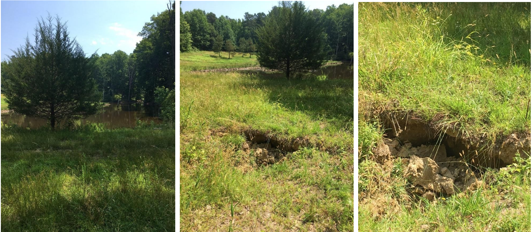
Figure 5: Site photos from COLO maintenance (On Mon, Jul 3, 2017 at 7:30 AM, William McQuillen <william_mcquillen@nps.gov>, COLO Yorktown Maintenance). Since these photos COLO maintenance dumped two loads of dirt in the hole. The dump material sank and a 20 foot depression formed around the hole.
