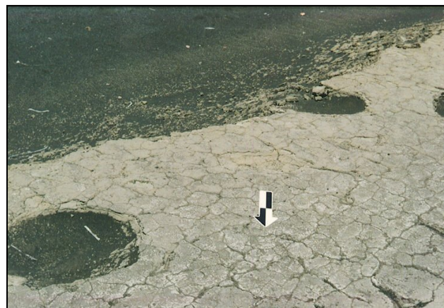
Photograph of ARPA violation in Area 2. Photo courtesy of Hawai'i Volcanoes National Park.
