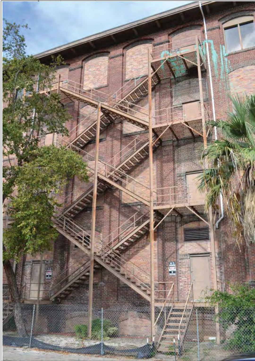
Figure 10. Main Mill, west façade, detail of fire escape that has been removed, 2007. Image courtesy of Wecco Development, LLC.
