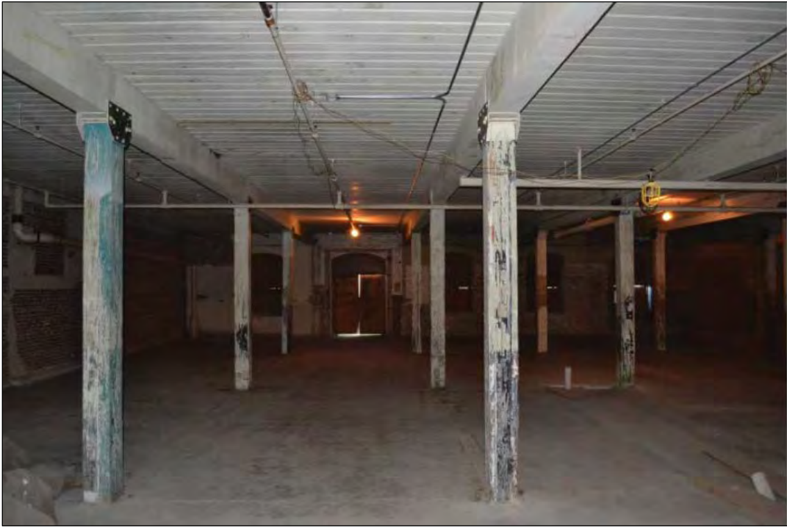
Photo 20: First floor, Building 8, looking east. Chamfered corners on posts and absence of a ceiling are both elements of slow-burn mill construction. Photograph by Wecco Development, LLC, 2013.
