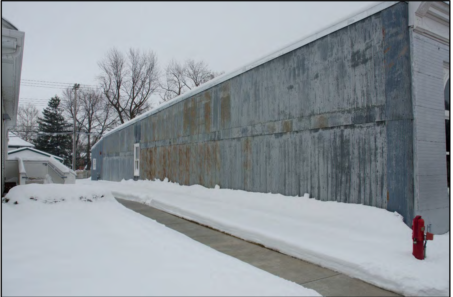
Photograph 4: KREGEL WINDMILL COMPANY FACTORY Nebraska City, Nebraska Exterior, west side; view northeast Photo by David Calease, January 2021
