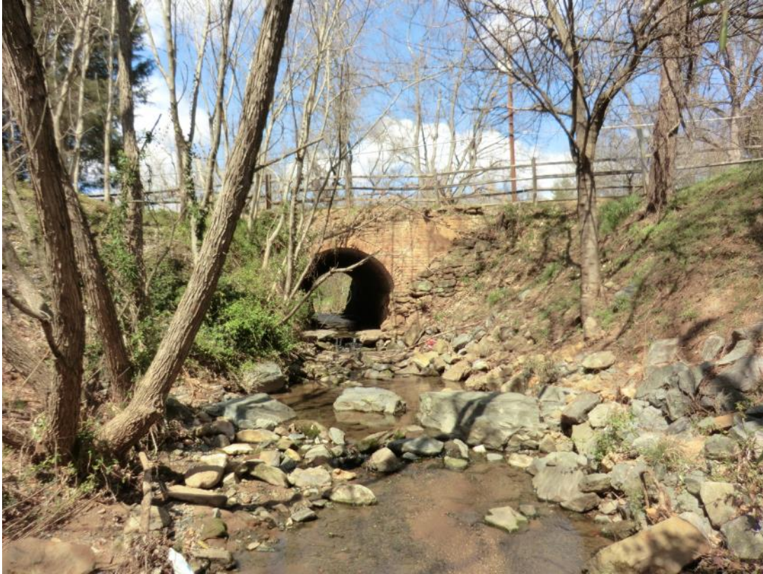
Brick barrel vault bridge over Tanners Run at Academy Street, looking north. Martha B. Hartley Photographer, April, 2013
