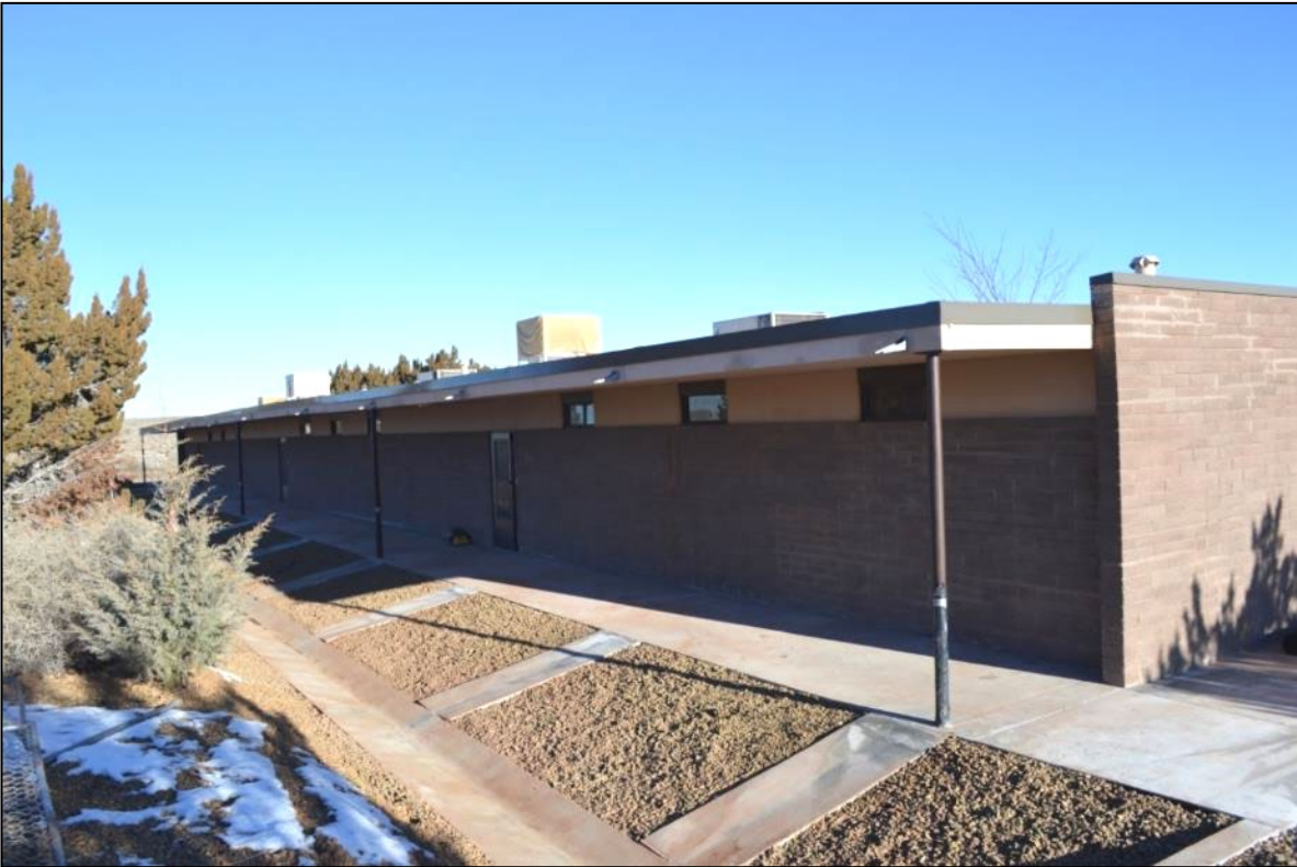
Photograph 25. Residence Block A (Resource 13), front (south wall) and part of east wall with 2016 drainage improvements in foreground.
