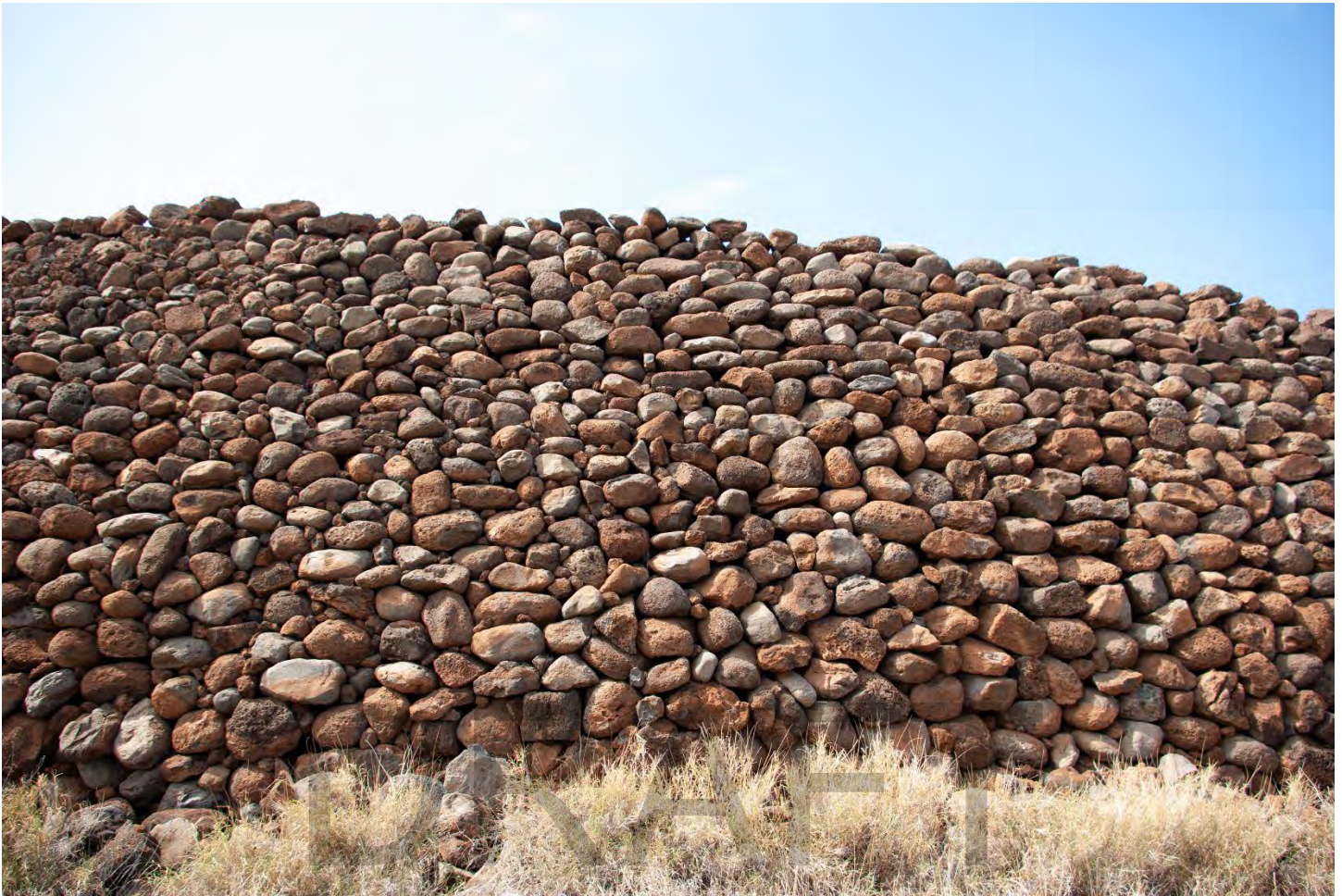
Photo #18 of 81 (HI_Hawaii_Puukohola Heiau NHL_0018) Pu'ukoholā Heiau, east wall. Camera facing west.
