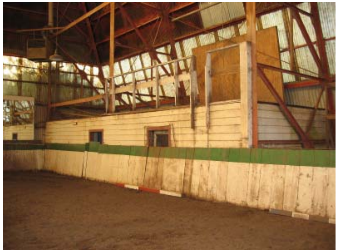
The southwest interior corner of the Balloon Hangar shows the original vertical trusses, rooms built during the Nike Assembly use of the building, plus the wall of the current indoor riding rink. (John Martini, 2003)
