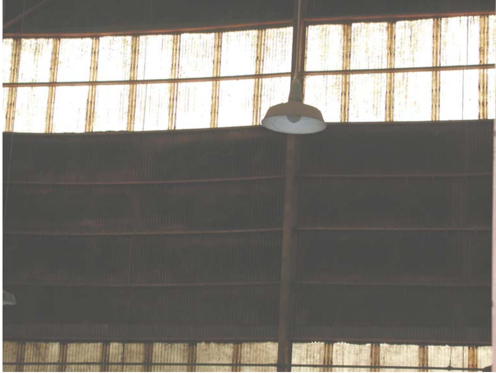
Sagging Wind Girts at South Wall
