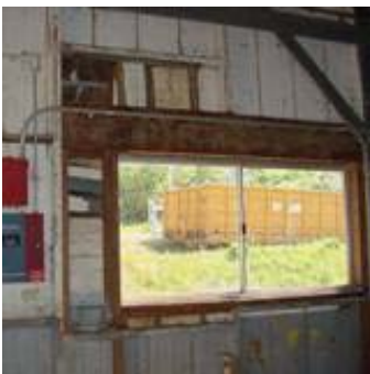
Sliding doors hanging from overhead tracks on West Vehicle Shed. (Jane Lehman, 2004)
