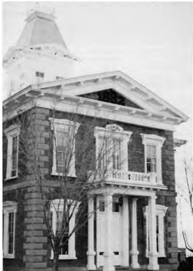
Tombstone Courthouse in need of stabilization. Photo by Jim Garrison, office of the SHPO, Arizona State Parks.
