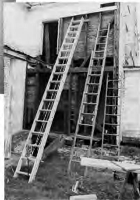
Mumma Farm House, Antietam National Battlefield, MD. A former window location was discovered during the removal of interior plaster. This feature should be recorded prior to the replastering of the wall surface. Photos by Thomas Vitanza, Williamsport Preservation Training Center, National Park Service, 1992.
