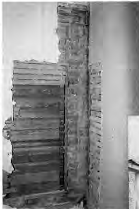
Mumma Farm House, Antietam National Battlefield, MD. The braced frame of the structure was discovered while siding repairs were underway. Drawings and photographs were made to document the framing system before the siding was replaced.
