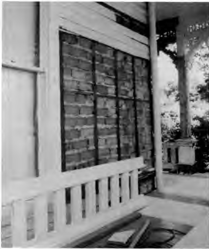
Figure 2. Cavity wall brick infill or "nogging" on the Truman home. This unique element would be sacrificed if insulation were to be installed. Photo by the author.
