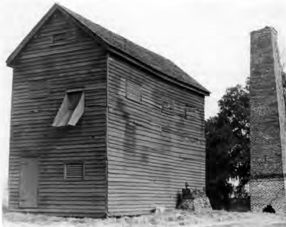
The rice barn and threshing mill at Mansfield Plantation, SC, were common features of Georgetown County rice plantations. Photo by Wyndell Peacock.
