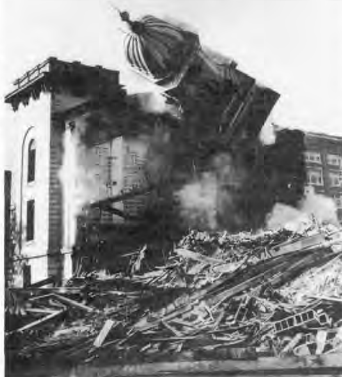
The 125-foot tower of the Lycoming County Courthouse in Williamsport, PA, falls during the 1969 demolition of the 109-year-old landmark. AP Wirephoto, RGW 51430rgw.
