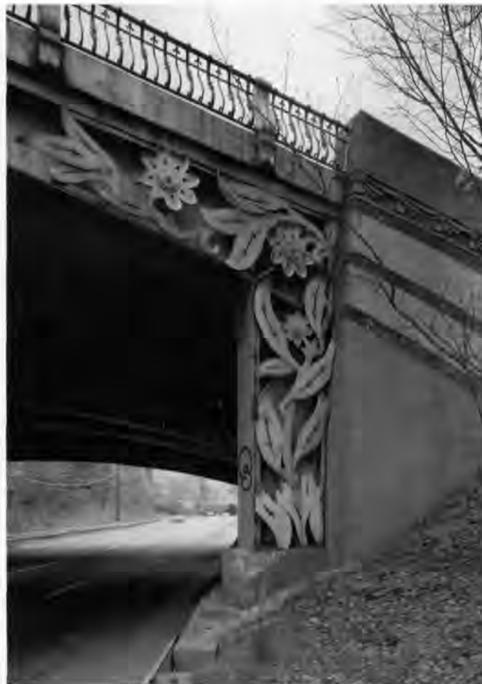
Detail of Main Street Bridge wingwall, constructed 1940, Merritt Parkway, Trumbull, CT. Photo by Jet Lowe, HAER.
