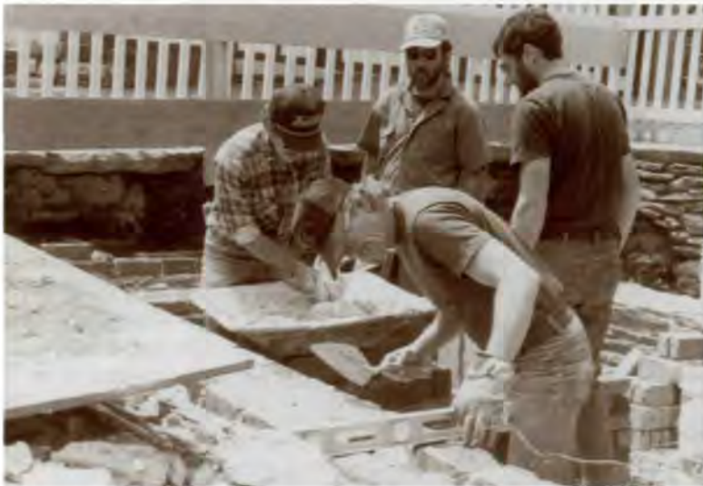
Masons from WPTC and the Southeast Preservation Crew participated in the reconstruction of the Burton Jewelry Store foundation.
