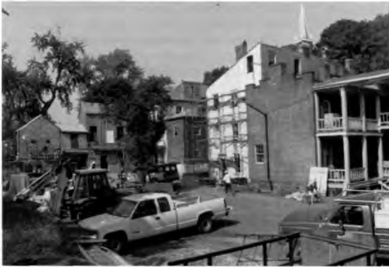
Package 116, Sept. 1995. Construction work in progress on buildings 32, 33A, 33, 34A, 34, 35, and 36, Lower Town.
