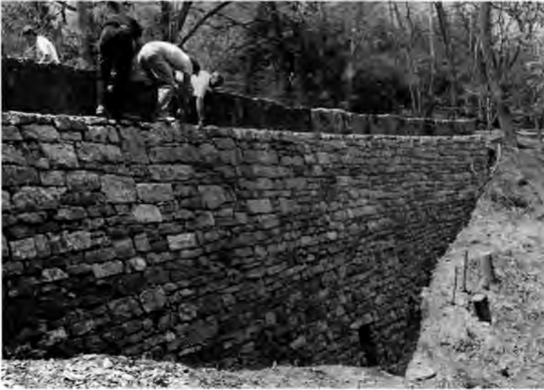
The park wall was completely dismantled and authentically rebuilt at a savings of $100,000 over the bid for a concrete replacement.
