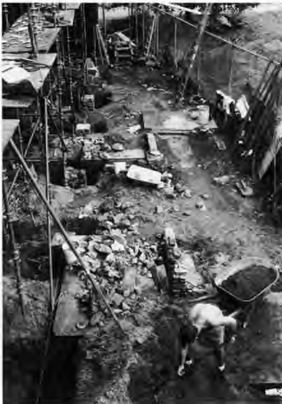
Interns assisted with the restoration of the Bowling Alley at Lyndhurst, Tarrytown, New York. Volunteer and internship programs get outsiders involved in a constructive manner beneficial to all parties. Photo by David Overholt.
