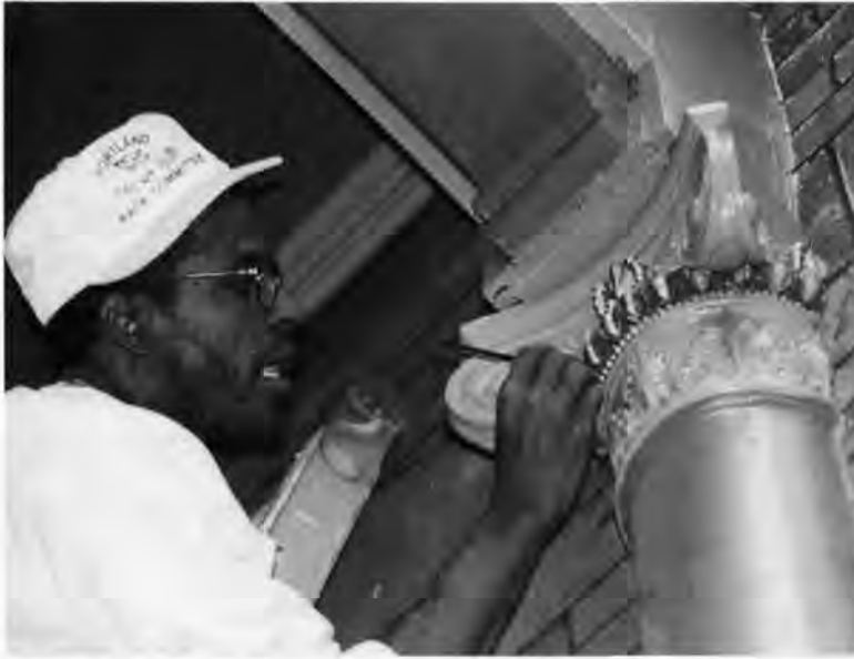
Shabazz, a painter, applies goldleaf to an Ionic column capital as part of the restoration project in New Haven, Connecticut.
