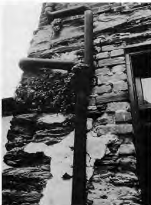
Minor repair deficiencies, such as vegetation growing out of masonry and leaky roof drainage systems, should be accomplished while in the field; either approach, "toolbelt" or "free-range" could perform the required task and contribute to the preservation of the building. Photo courtesy HPTC.
