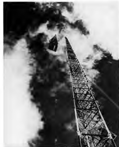
Historic photo of BREN tower under construction courtesy U.S. Dept. of Energy.
