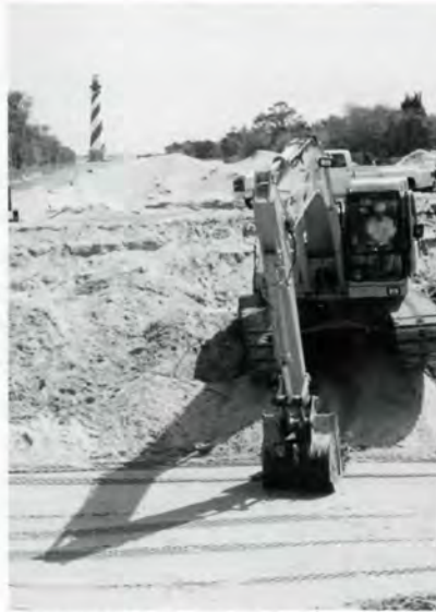
Preparing the new site to receive the tower. Photo by Steve Kozosky.
