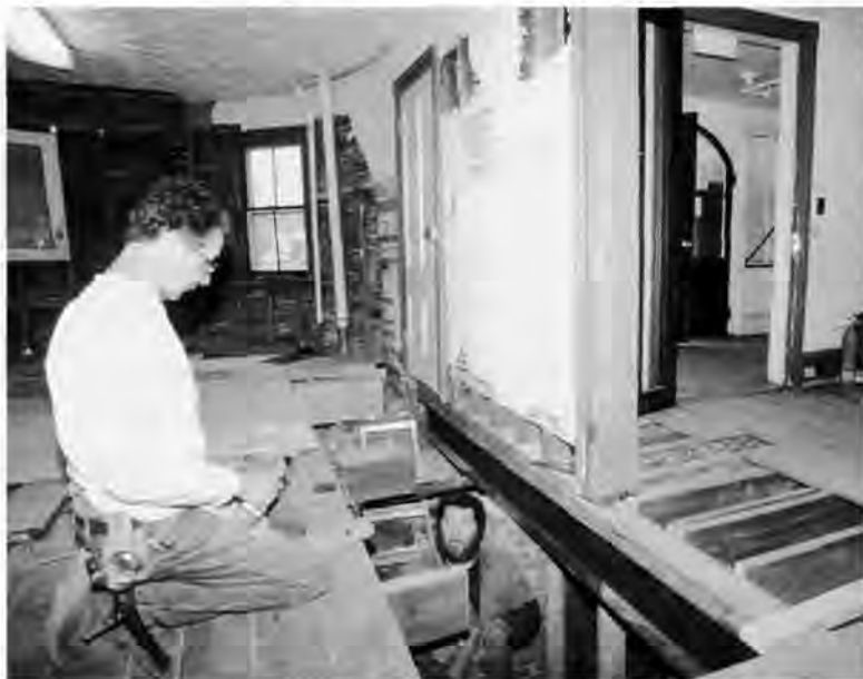
The crew of structural repair subcontractor H.R. Bixler installs a steel girder below the interior bearing wall partition separating Peirce's parlor and study.
