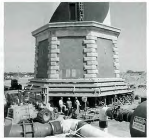
The lighthouse tower on a temporary support system. Note one of a series of sensors (at right on tower base) which will be connected to a central monitor to direct the operator to adjust the hydraulic jacks that will support the tower during the move. Photo by Steve Kozosky.
