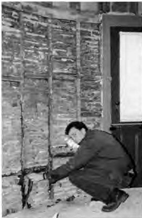
Peirce's former study during destructive investigation. Exhibit Specialist Paul Jaeger points to decaying exterior wall framing damaged over the years by moisture wicking through the riverstone veneer installed by Peirce in 1909.
