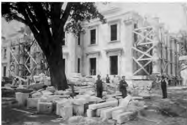
The Vanderbilt Mansion under construction in Hyde Park, New York, 1895. Courtesy National Park Service.
