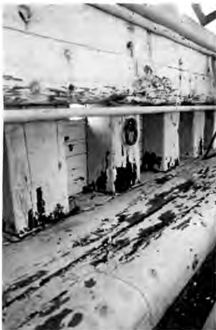
Dry rot in the bulwark, stanchions, and waterway of Wapama . (Photo courtesy of National Park Service/Richard Frear)
