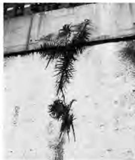
Plant growth left unattended will gradually enlarge the crack in this wall, and result eventually in spalling of the stucco, which may require extensive repair.
