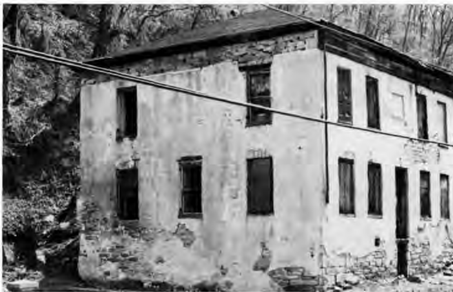
Patches of stucco have fallen off this 19th century building exposing the rough-cut local stone substrate. The method of building construction revealed by the missing wood entablature on the side indicates that the building was stuccoed originally, and most likely scored in imitation of ashlar masonry.
