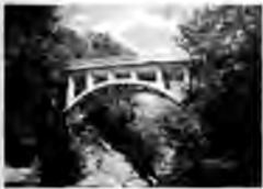
FIGURE 3 This open spandrel concrete deck arch carrying Route 30 over Mine Kill in Schoharie County was included in the field review and was determined to be eligible for the National Register. (Courtesy of Mead & Hunt, Inc.)
