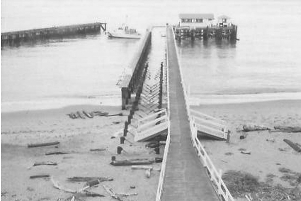
History figure 9. Photograph of deteriorated marine railway in 1978 shortly before its complete demolition. Photograph taken by Gordon Chappell—PWR Historian. [45]
