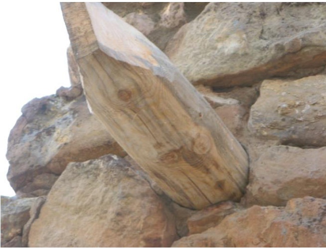
Complete replacement, "beaver cut" end
