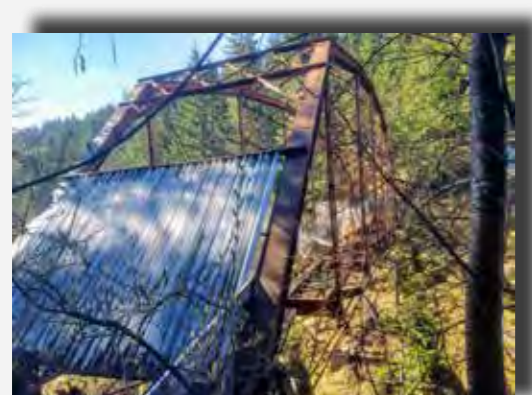
Bridge with barrier and lack of decking
