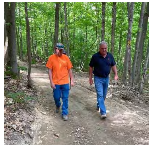
Gregory Muller, NYSDEC West Almond supervising forester, and contractor Tim O'Rourke inspect the construction on Trail 4 in 2022.
