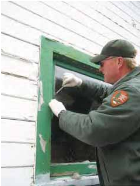
A historic preservation crew member performs delicate work to restore a window on the historic Lifesaving Station, a national historic landmark. PHOTO BY KRISTIN GILLISS
