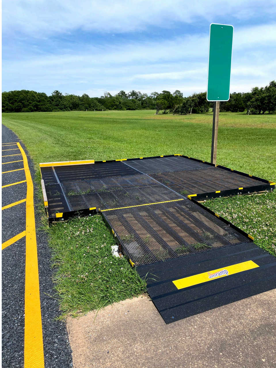
Figure 8: Accessible Ramp and Platform Installed at Sculpture Stop Source: U.S. DOT Volpe Center
