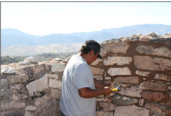
Figure 4: Preservation Mason removing portland cement by hand to preserve the original fabric of the wall. Photo NPS
