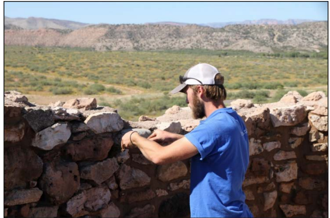
Figure 5: Preservation Intern replacing historic concrete mortar with soil cement to stabilize the wall. Photo NPS
