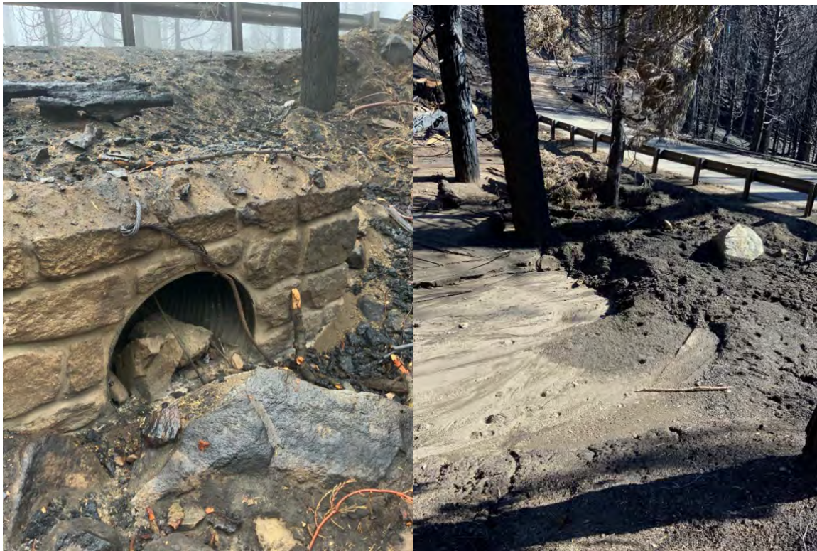
Figure 1. A culvert up the road from Red Fir Maintenance facility before and after the Oct 25 storm
