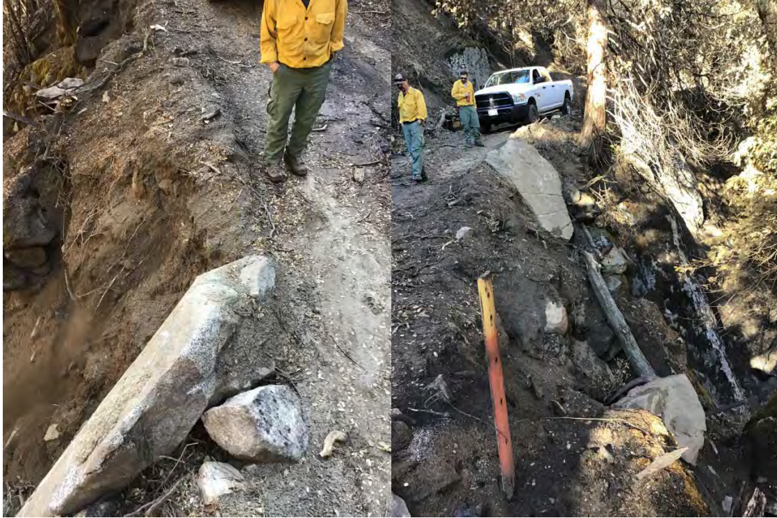
Figure 2. Oriole Lake road retaining structure lost
