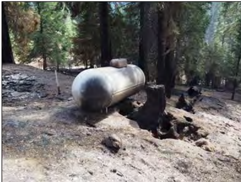
Photo 3 Redwood Mountain Ranger Station propane tank. View looking southeast.
