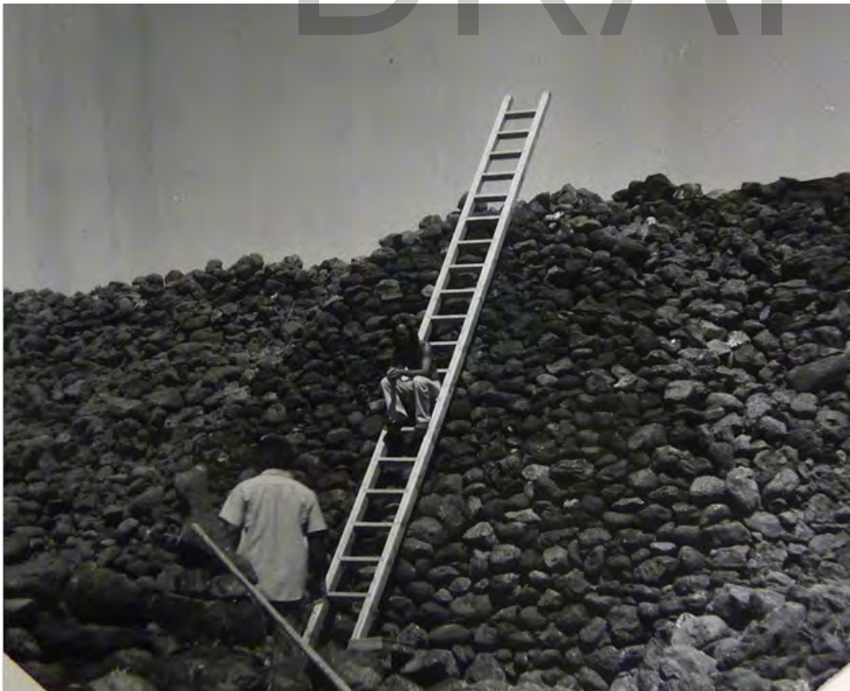
Figure 37. Emergency stabilization of Pu'ukoholā Heiau during the 1970s. Photograph courtesy of NPS
