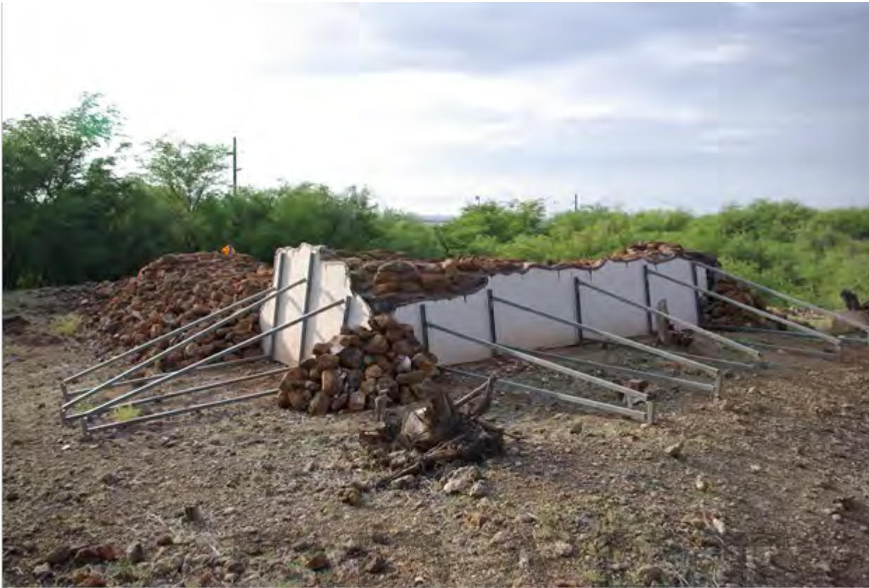
Figure 43. John Young's primary residence at the John Young Homestead. Steel bracers and cement board siding protect original portions of the eastern and southern walls from the weather. View to the northwest.
