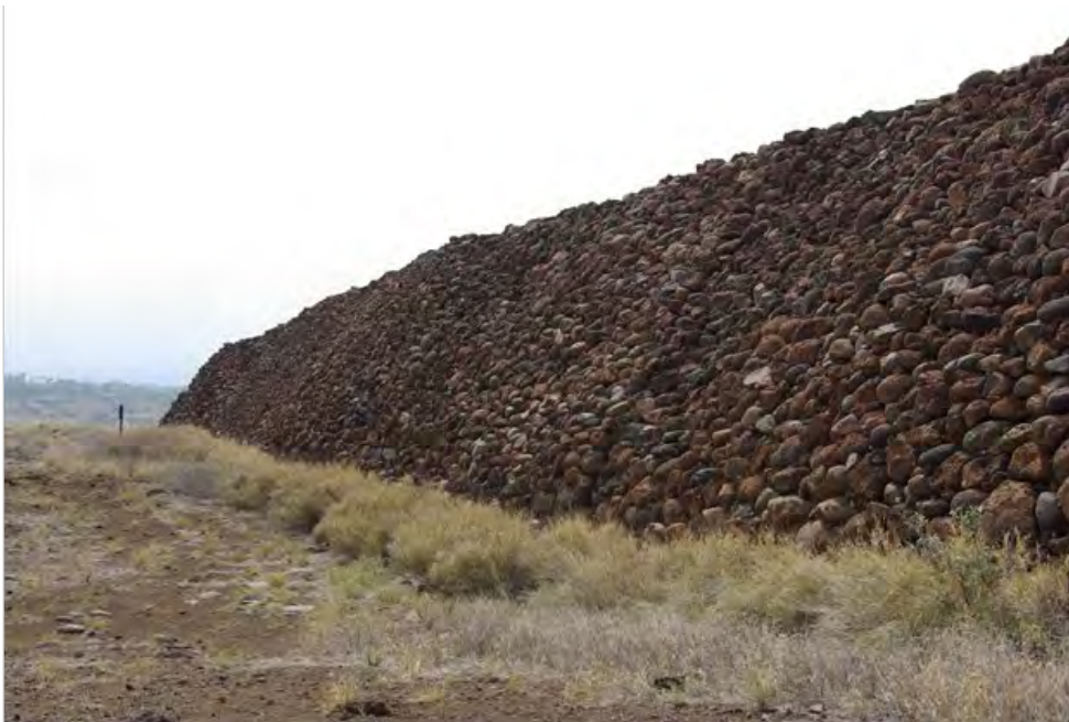
Figure 40. The east wall of Pu'ukoholā Heiau. The vertical bulges in the wall were formed during the 2006 earthquakes. Photograph courtesy of NPS.
