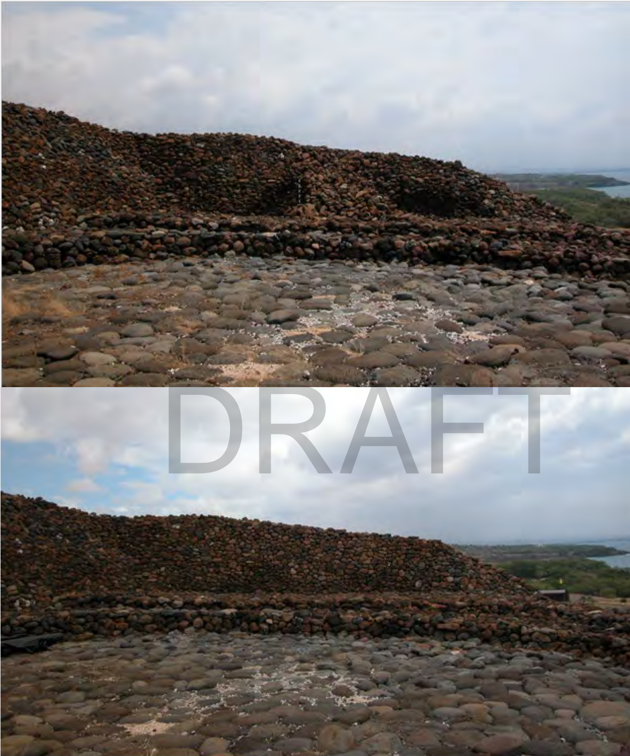
Figure 39. Comparative images of a wall in the southern section of Pu'ukoholā Heiau, showing damage caused by the 2006 earthquakes (top), and repairs completed during emergency stabilization efforts (bottom). Photographs courtesy of NPS.
