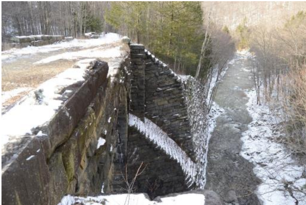
6. Buttresses and revetment/retaining wall at north corner of Bridge No. 6, looking northwest. John Daly, PAL, 2017.
