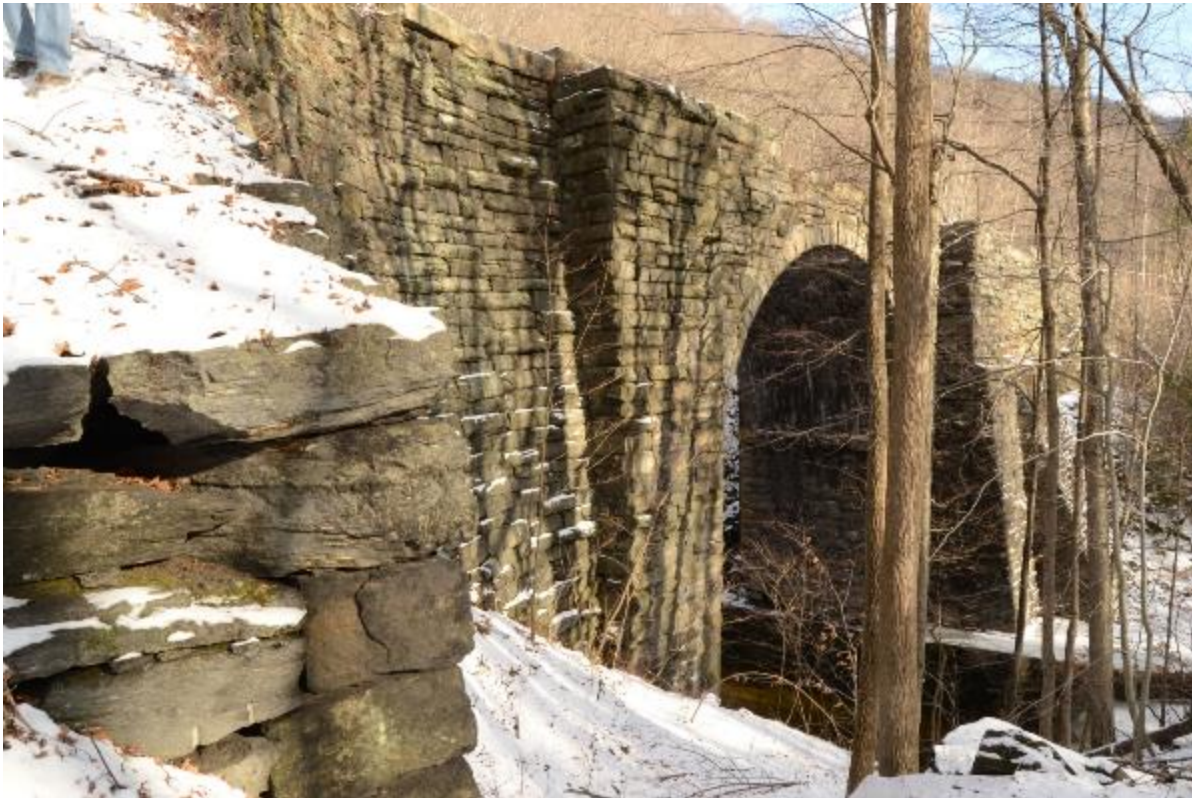
2. Oblique view of southwest (downstream) elevation of Bridge No. 6, looking east. John Daly, PAL, 2017.
