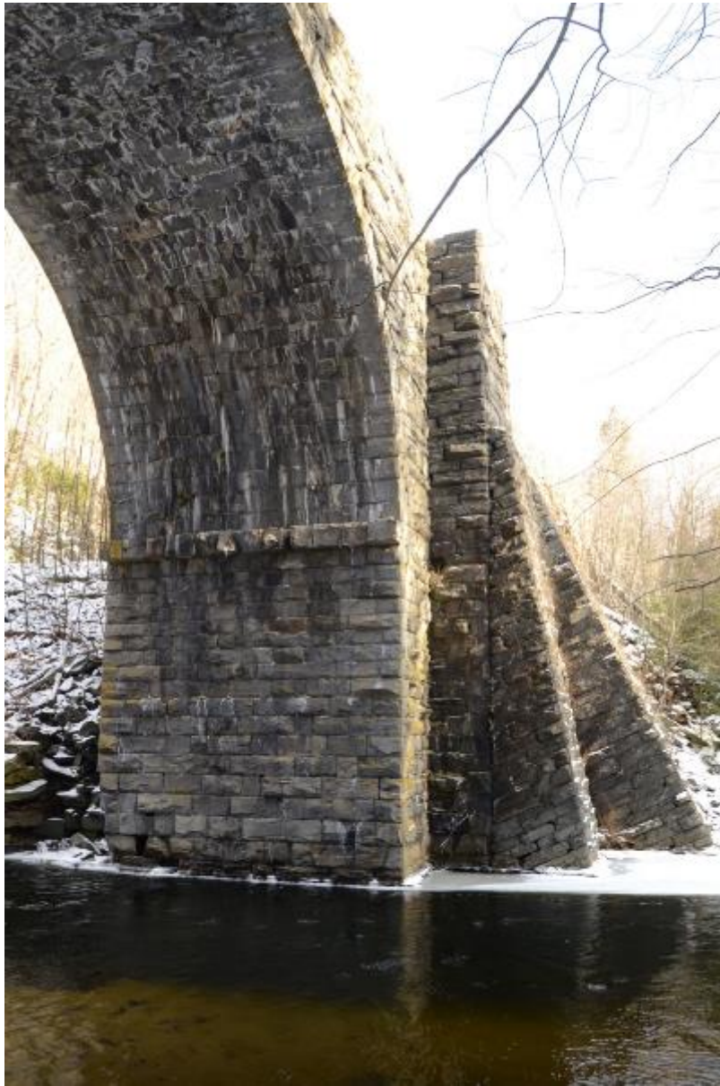
4. Southeast abutment and buttresses of Bridge No. 6, looking east. John Daly, PAL, 2017.
