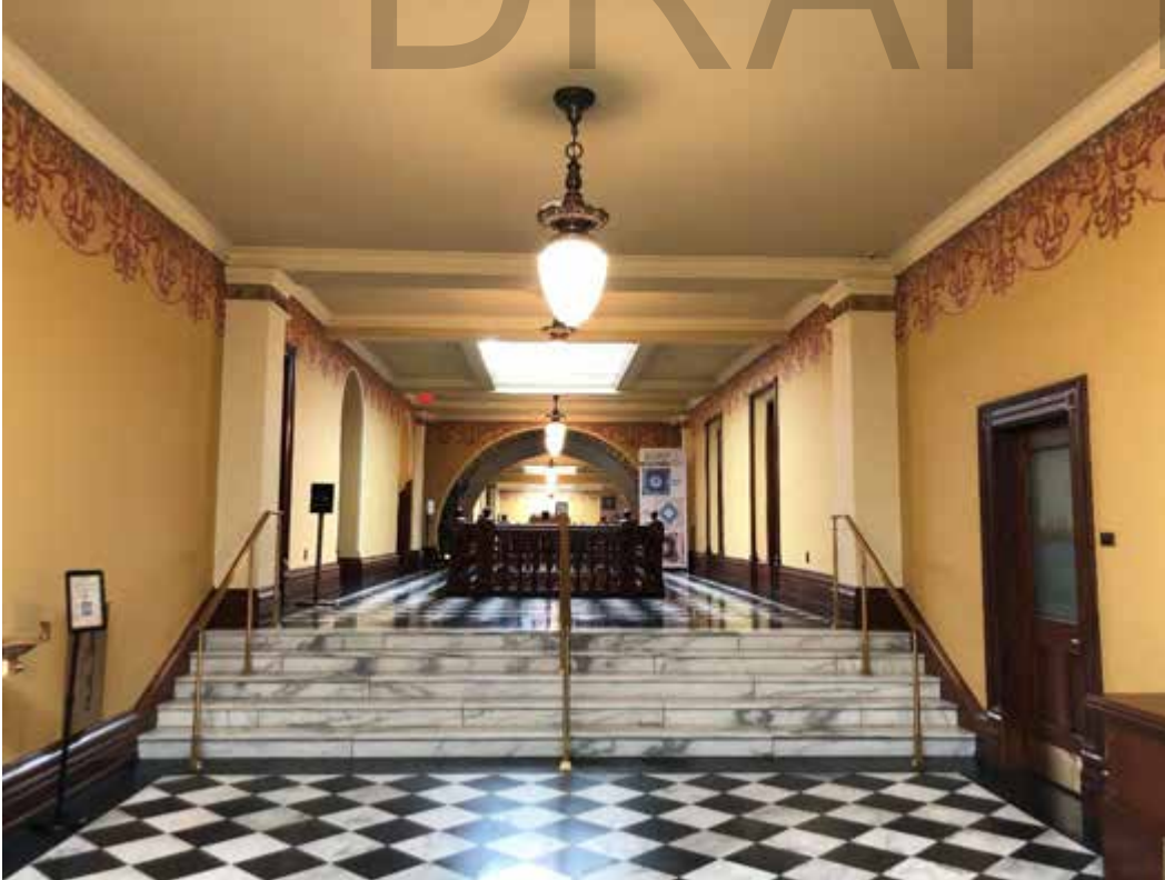
Photo 29 of 55: Third-floor hallway looking toward rotunda. Stairs leading to 1890 wing in foreground. Note balustrade surrounding lightwell and restored laylight above. May 2021.
