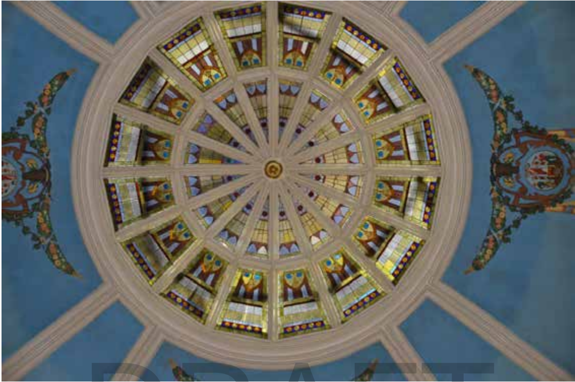
Figure 37: Rotunda ceiling and laylight prior to 2019 restoration. (Wyoming Capitol Square Project/ http://www.wyomingcapitolsquare.com/ )
